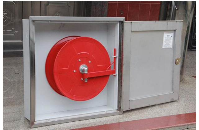
Stainless Steel Fire Hose Cabinet
